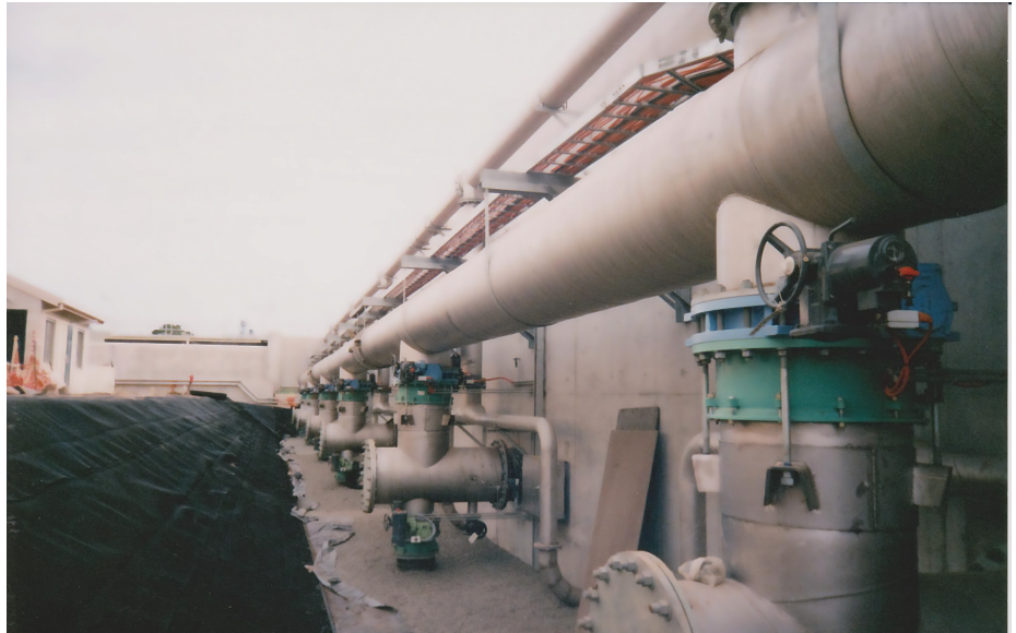
Appin Sewerage Treatment Plant, NSW. Fabricated and installed by ASSDA member and Accredited Fabricator Roladuct Spiral Tubing Pty Ltd using 316 grade stainless steel. Image courtesy of Roladuct Spiral Tubing Pty Ltd.
